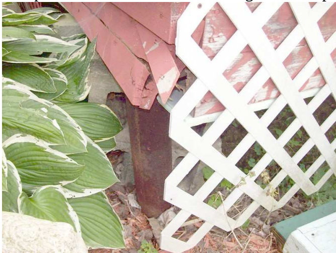
This pipe column is no longer plumb and vertical. The column has damaged the supporting materials. The concrete blocks, utilized for temporary support, are not on proper footings and are no longer stable in supporting the load.
