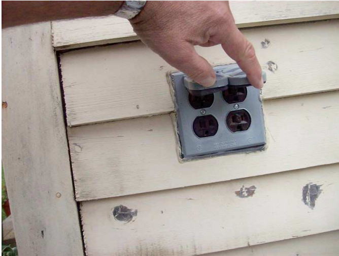
The exterior outlets are not protected by Ground Fault Circuit Interrupters (GFCI).
