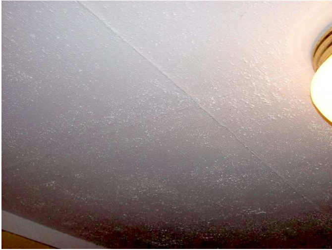
The ceiling in the bathroom is poorly finished and should be repaired.
