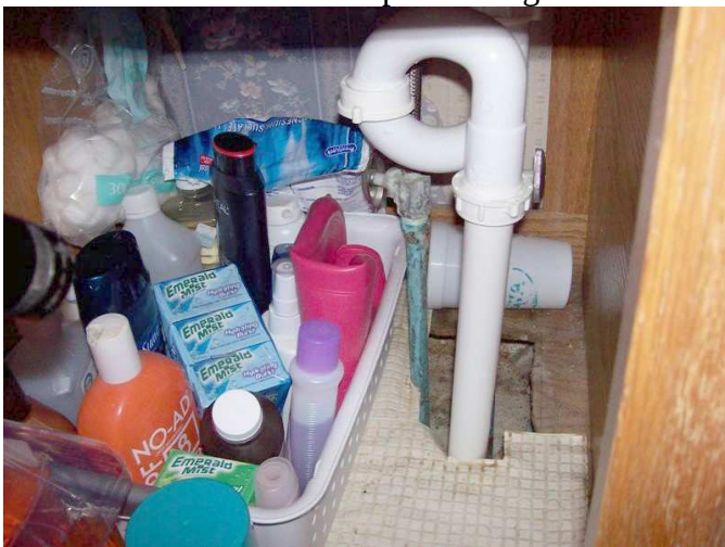
Under the bathroom vanity in the laundry area the water supply piping has had a leak and damaged the floor of the cabinet.
