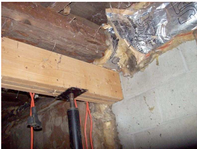
This system of repairing a beam is not correct. The new beam is not tight against the existing beam, not anchored to the wall, and not bearing on a proper masonry pilaster. It is also important to note that the column is not anchored to the beam and the new beam is not anchored properly to the beam it is supporting.
