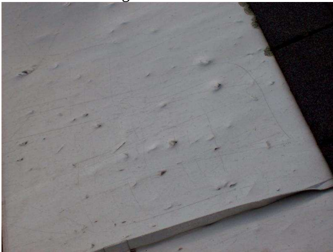
This is an additional photo showing the damage to the ice guard on the roof.
