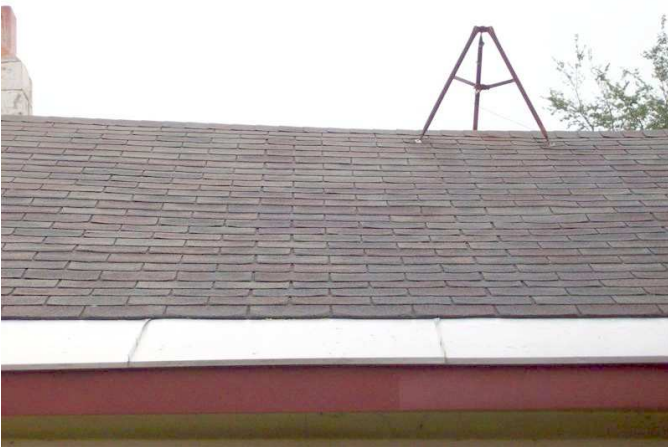
This photo shows the wavy roof surface. If the roof is stripped and replaced there may be some sub sheathing that will need to be replaced as well as some rafters should be reviewed. The roofing system has a very minimal ventilating system installed.
