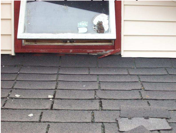
This photo shows a casement window has broken trim. It also shows some broken tabs of shingle on the roof.
