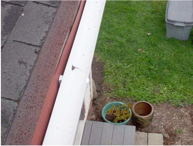
This gutter has a hole in it.
