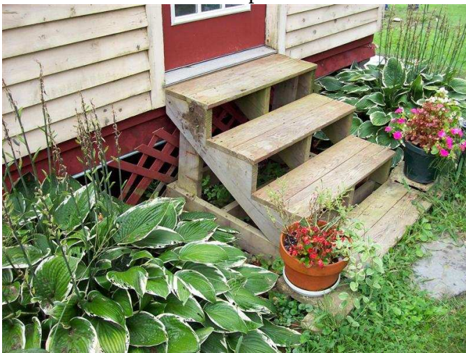
The porch stairs require proper handrails in an effort to prevent a fall.
