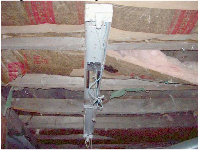
This light fixture in the basement should be removed if it can not be repaired.
