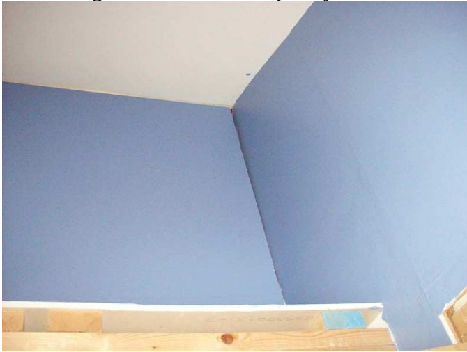
The interior of the dwelling has several locations where the corners of the sheetrock are not finished. There are openings for closets and interior doors not completed with trim.
