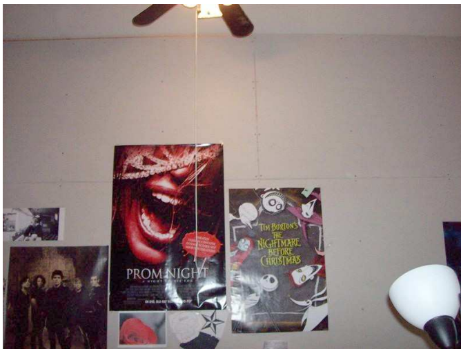
This wall is not finished with tape and sheetrock mud.
