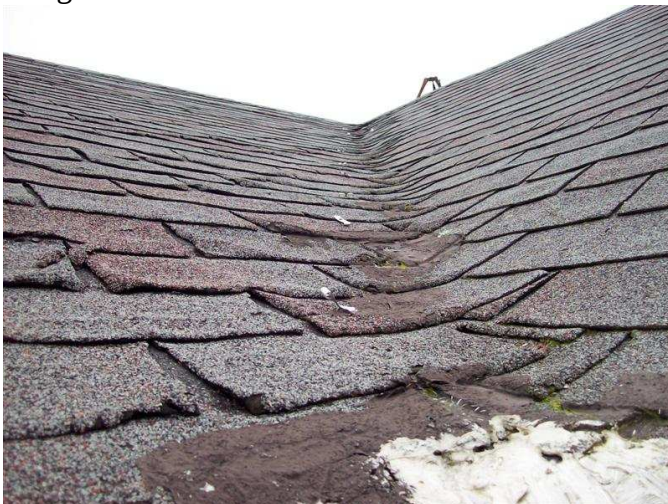
This is a view looking up the valley showing the very poor condition of the shingles.
