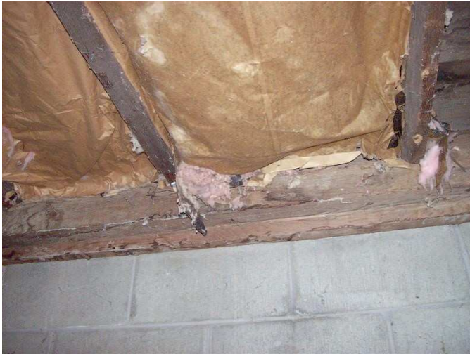
This photo shows that mice have been nesting in the insulation for the basement.
