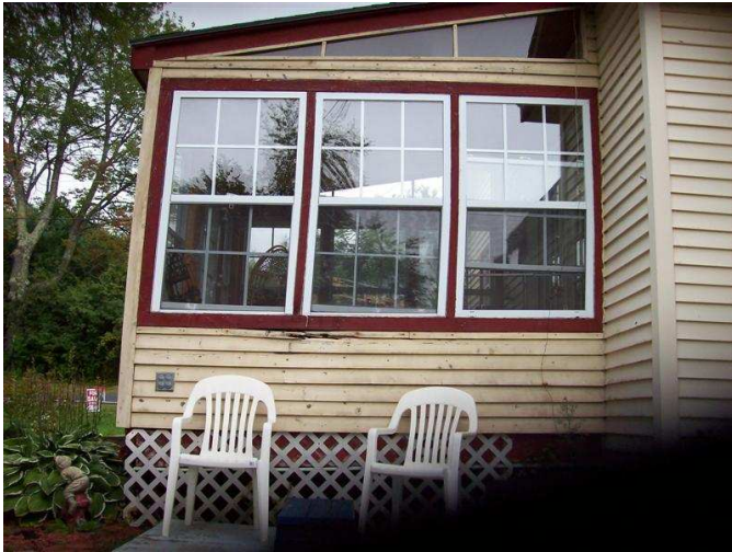
This photo shows the windows bowing under the pressure.
