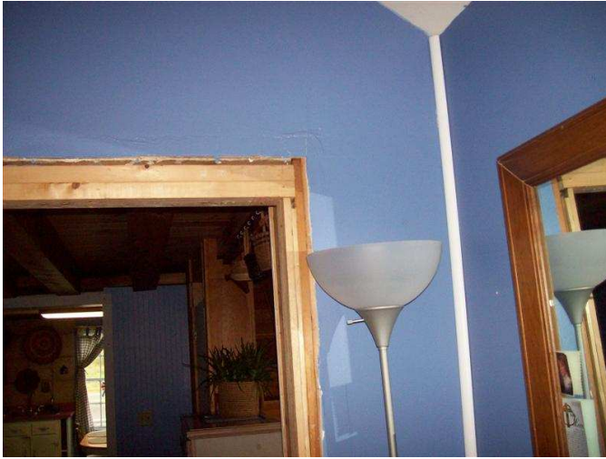
This door opening is not finished.
