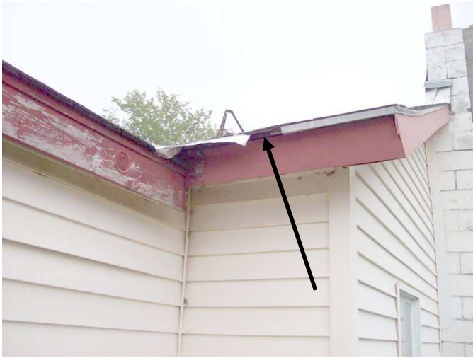
This valley flashing is not properly completed and the drip edge is not complete.
