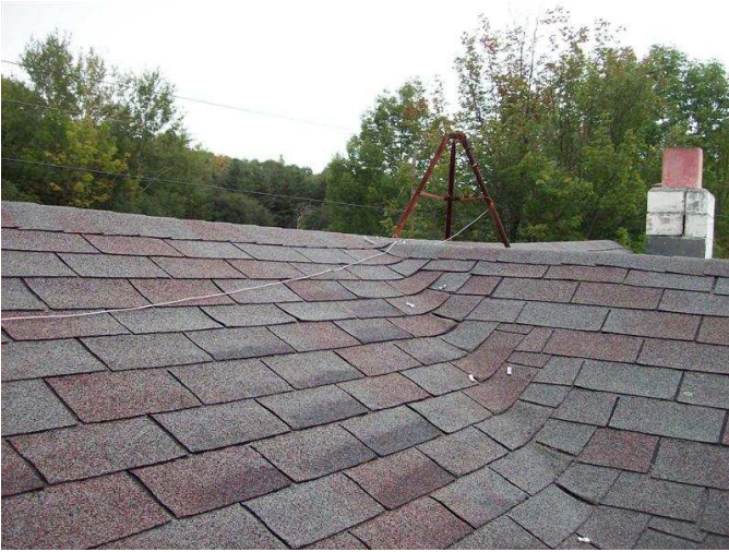
This photo shows the sag in the ridge of the main portion of the dwelling.
