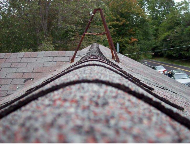
This photo shows a different view of the sag in the ridge. The sag may be from normal settling but could also be a sign of a deteriorated ridge. Very minimal ventilation is provided for the attic space.
