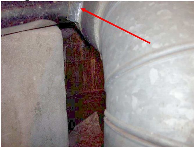
The connection of the hot water heater vent to the furnace vent is not properly installed. The connection should be by a properly installed thimble connection. Cutting a hole into the main vent and sticking the pipe into the hole could cause it to become blocked and back vent into the dwelling causing risks to health and safety.
