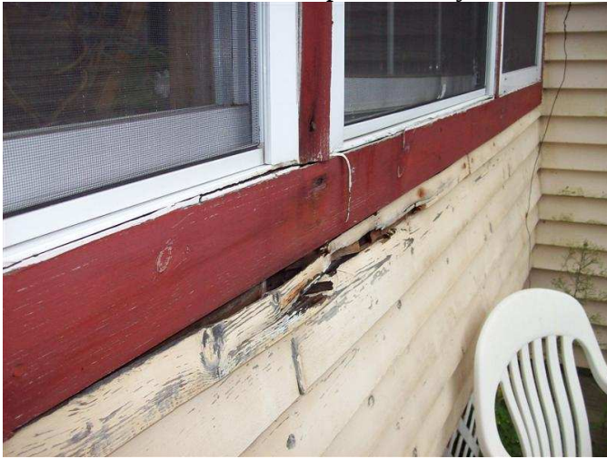
This is a closer view of the porch and the moisture damage.
