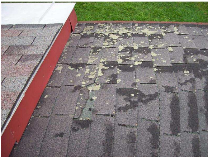
More broken shingles and some algae is growing on the roof.
