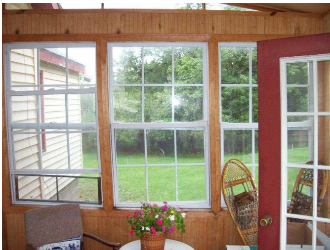
This photo shows the porch windows failing under the stress of the porch as it is settling. The window to the left will not close properly over the screen insert. It touches at the top on the left but not on the top on the right.
