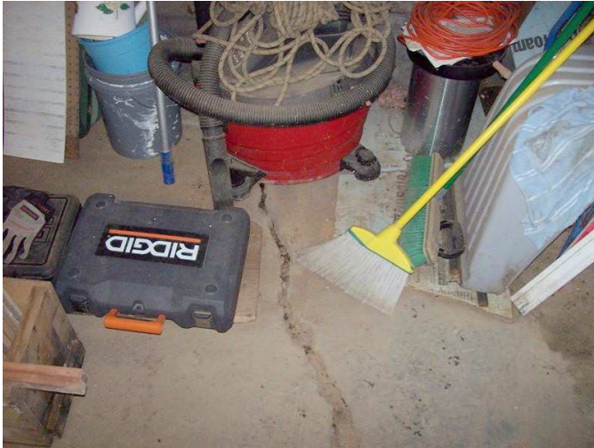
This photo shows the large settlement crack in the concrete floor.
