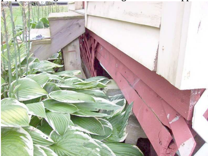
The damage to the porch is being transferred across the front of the entire porch.
