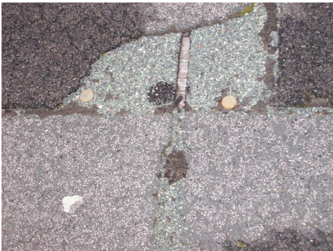
This photo shows the wood sub sheathing is showing through the roofing shingles as well as exposed fasteners.
