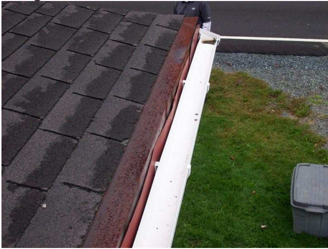
The metal fascia is not installed properly to protect the wood fascia from water damage.
