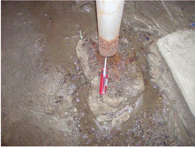
This column in the basement is rusted through and ready for replacement.
