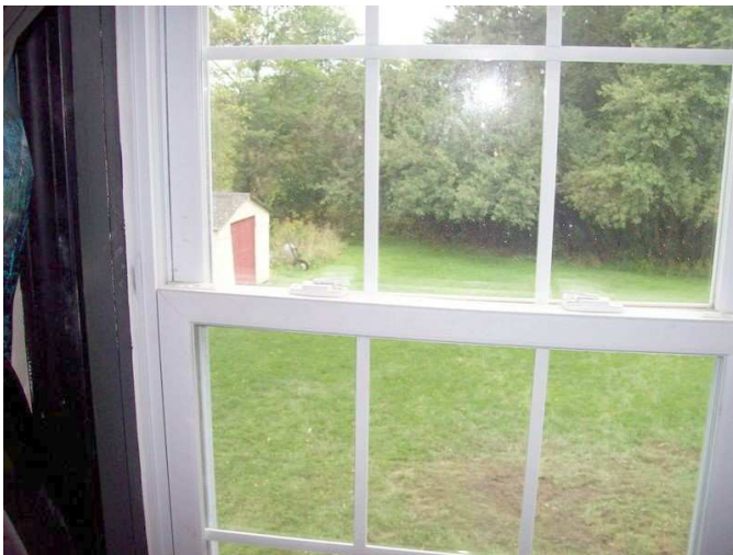
This window will not close as the window is not installed plumb and straight or there is settling in the exterior wall that is pulling the window casing out of plumb.
